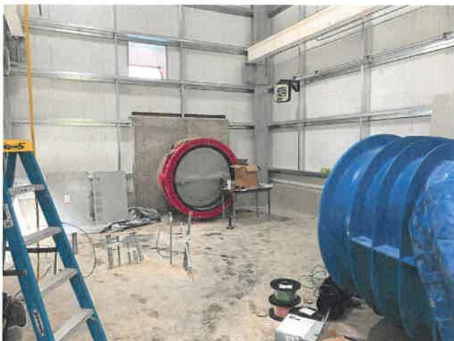
(Pictured above: penstock connection to the hydro turbine)
